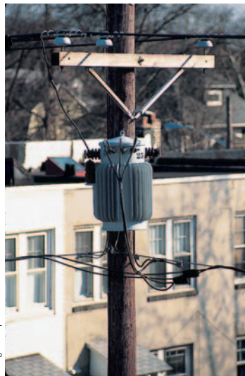
This cylindrical step-down transformer drops the voltage from 4 000 V to 220 V for delivery to a group of residences.
