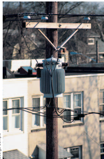
This cylindrical step-down transformer drops the voltage from 4 000 V to 220 V for delivery to a group of residences.
